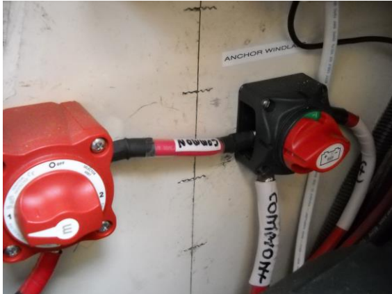
Picture of isolation switch in battery compartment
