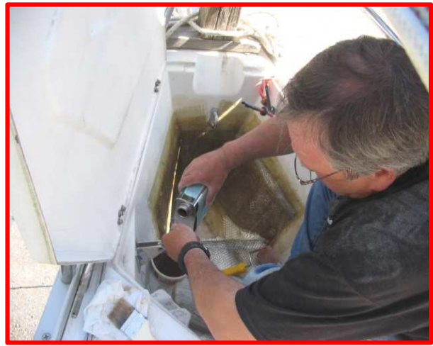
Using FB roving mat and resin, the chain locker walls were rebuilt to be as strong as original, and be able to accept 75' of chain and 150' of 3-strand 5/8 nylon rode.
