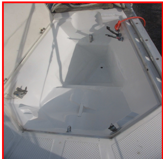
Painting completed, cover was then re-installed one more time for the final cutting measurements after frame and plate installation.
