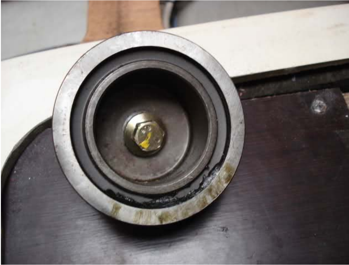
Worn and greasy idler close up
