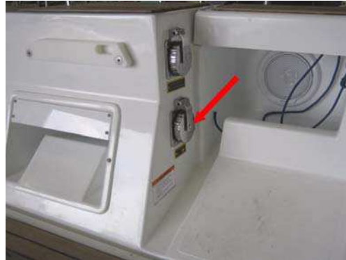
Shore power socket 220V - 32A (Ref 1)
