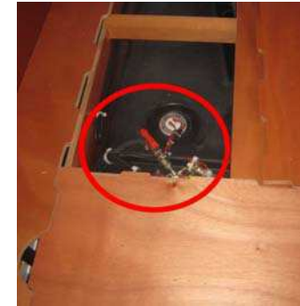
Supply valve Tank (Ref 1)
