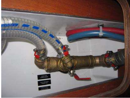
Sink drainage valve + Cooler Location: Under the sink
