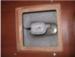
Electric bilge pump aft Location: Sump Capacity: 46 l / minute
