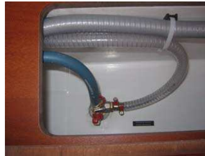
Seawater inlet / House water
