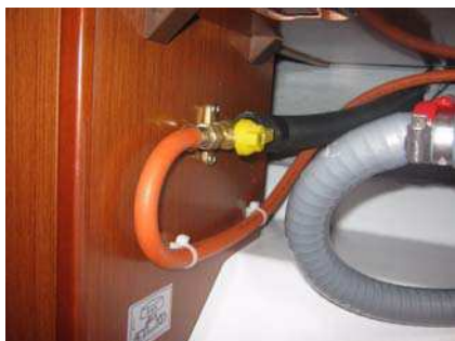
Supply valve - Gas
