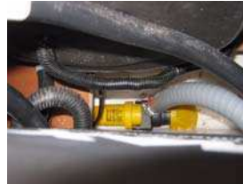
Forward bilge pump Location: Under - Bow thruster Capacity: 30 l / minute
