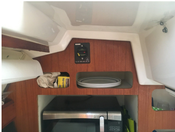
Breaker installed in Galley
