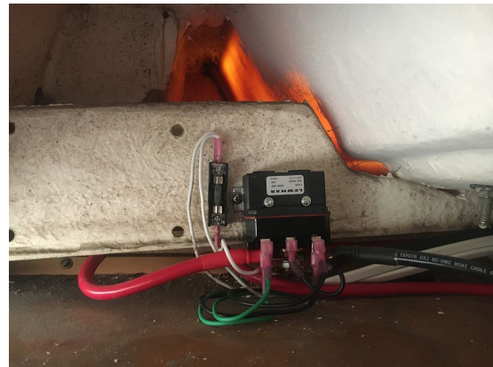
Contactor installed in starboard locker
