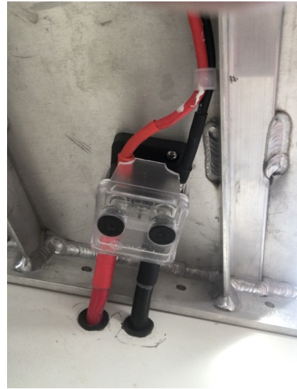
Electrical connection below support plate
