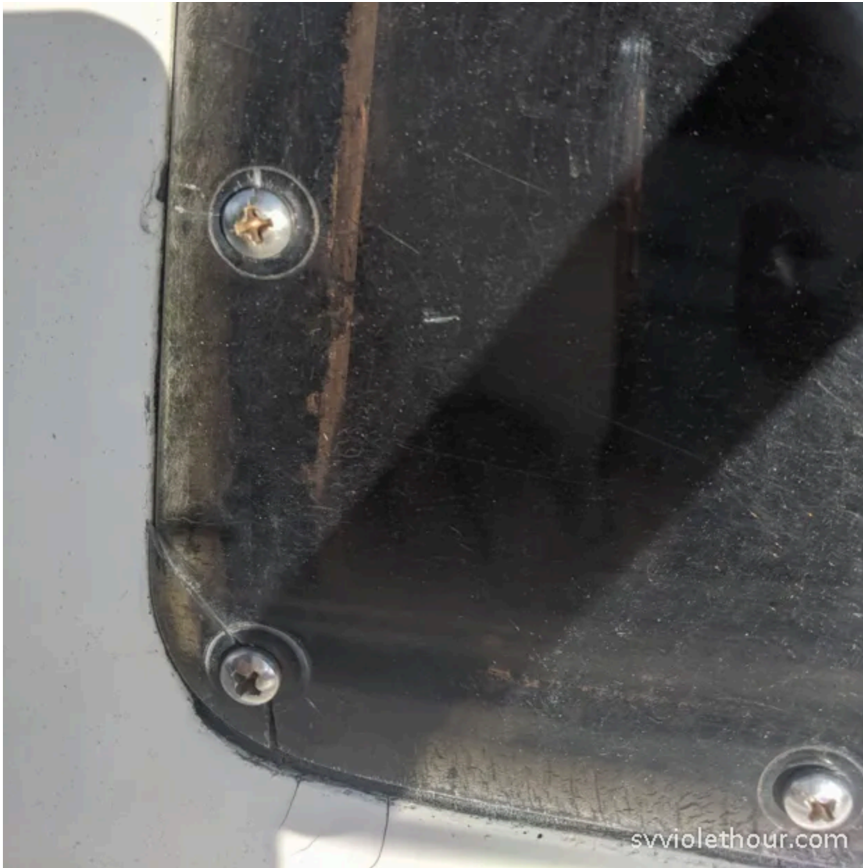
Old window with thru-bolting, cracked in bottom corner
