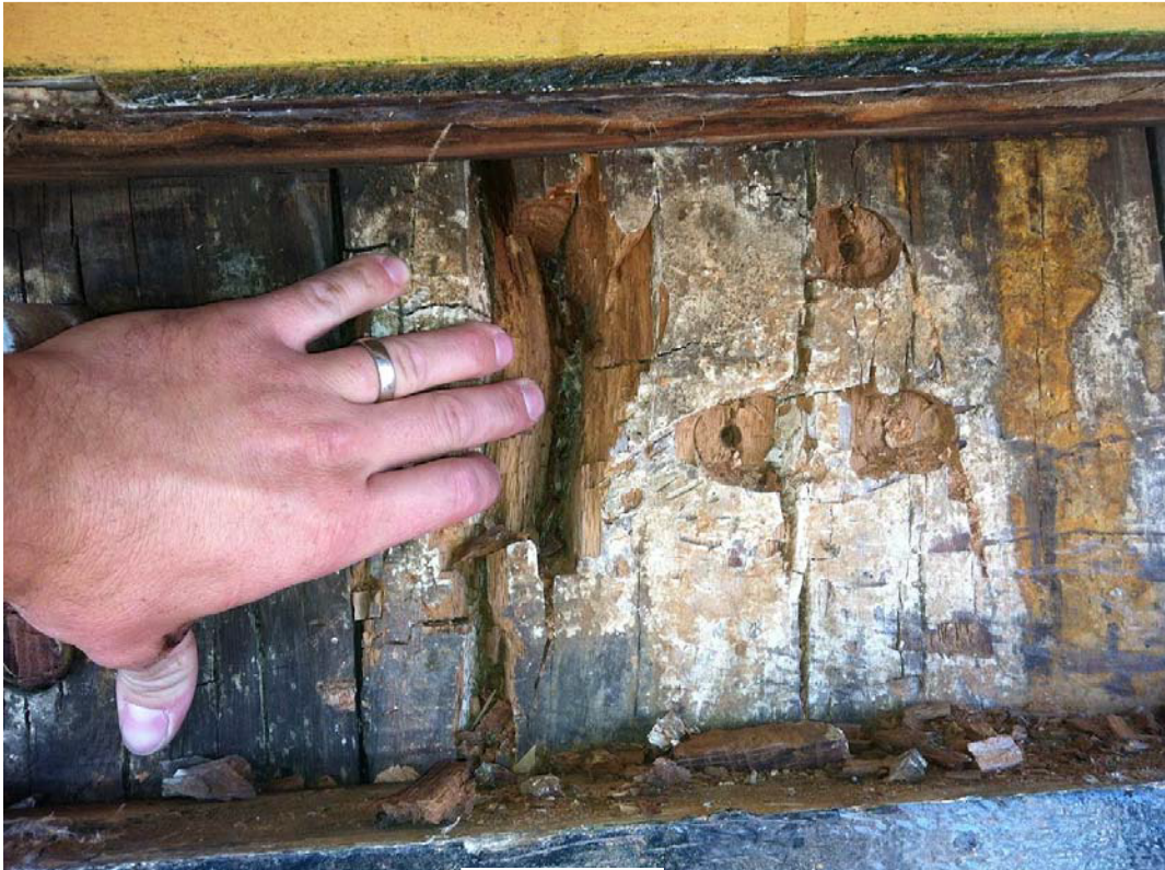
Figure 17 Photo of frame decay taken by [REDACTED].
