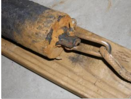
Detail of counter weight rope attachment point. The counter weight was sold for scrap. The table was easy to adjust without the counterweight.
