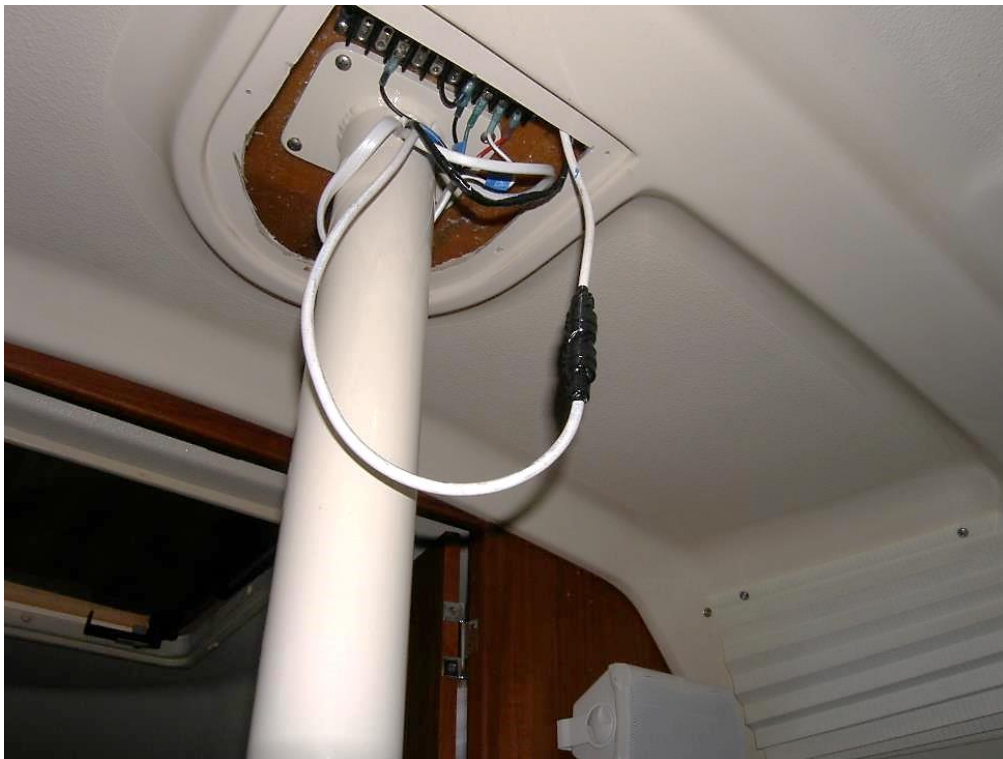
New mast wiring and VHF coax. Lightning ground runs through post down to keel bolt. Mast wires terminated in adhesive-lined shrink ring terminals. New coax connector wrapped in electrical tape. Should have used self-fusing tape.
